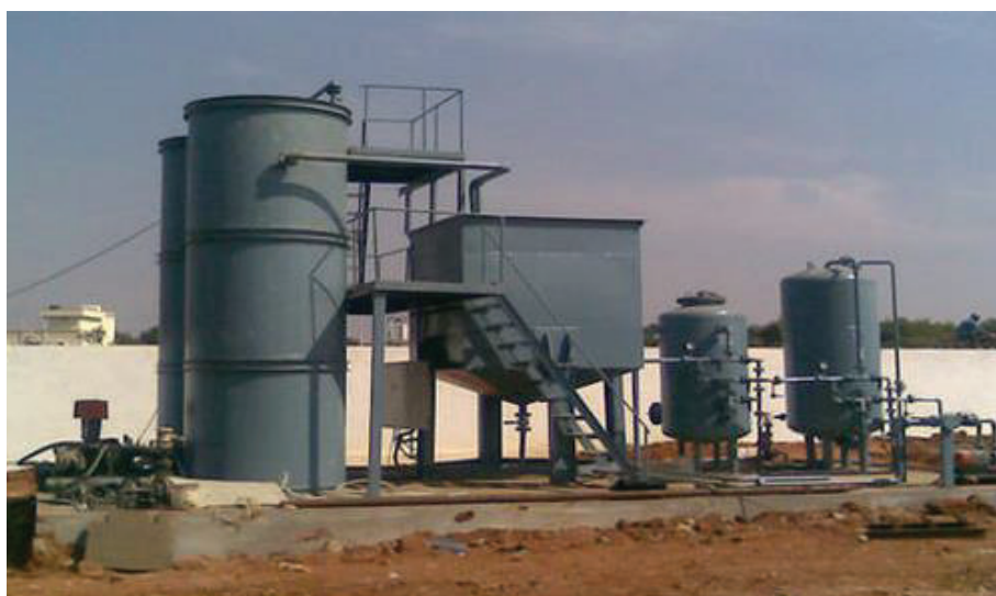
FIGURE 27: PICTURE OF A MBBR WASTEWATER TREATMENT PLANT (FOR REPRESENTATION PURPOSE ONLY; NOT TO THE SCALE)
